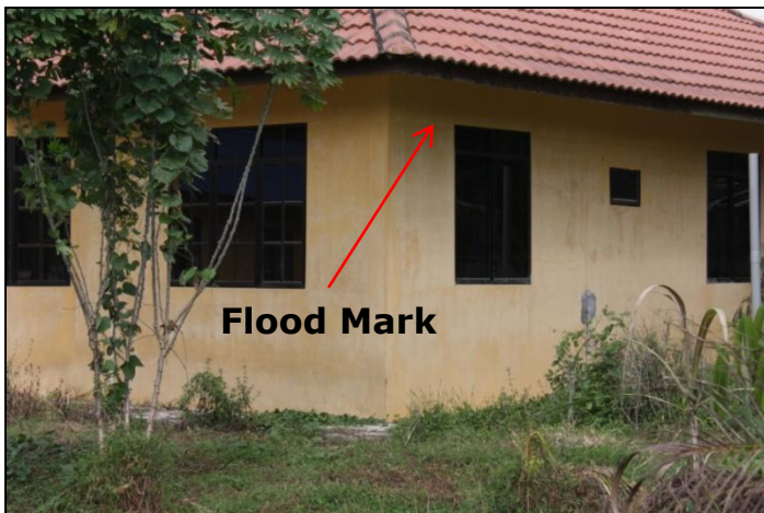
Flood Prone area at Kg Kundang Ulu
