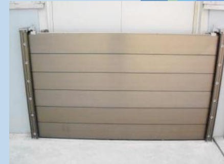
Metal Floodwall, China
