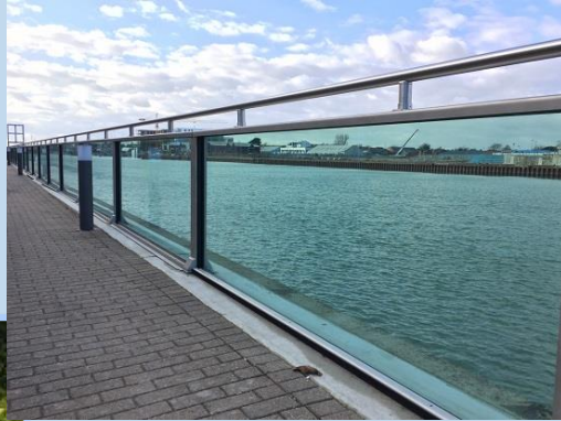
Glass wall barrier, Shoreham, UK
