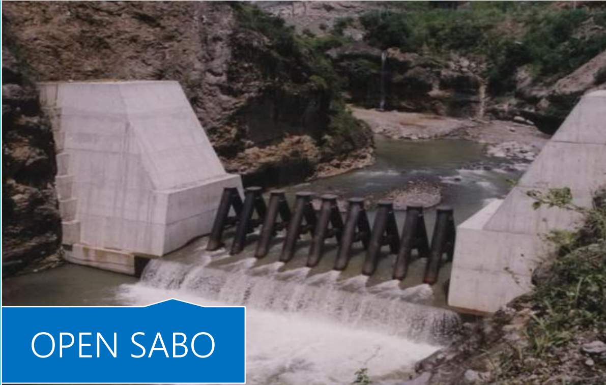
Open Sabo (Segawe) located in Indonesia
