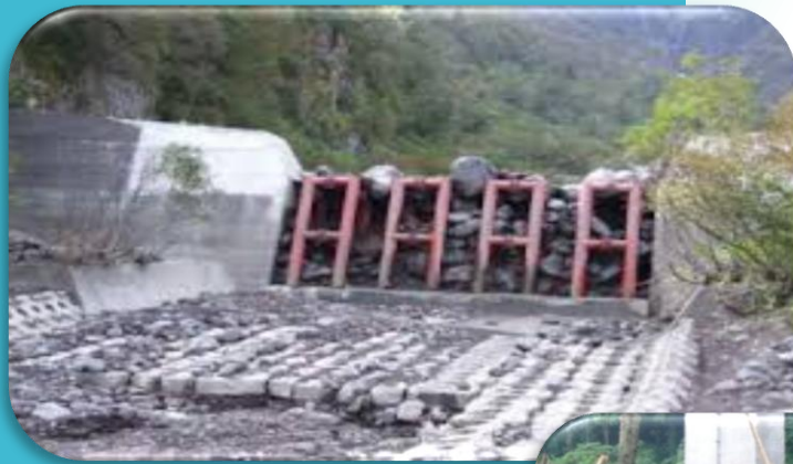
Sabo Infrastructure at Hokaido, Japan Source: Sabo & Landslide Technical Center, Japan (2019)
