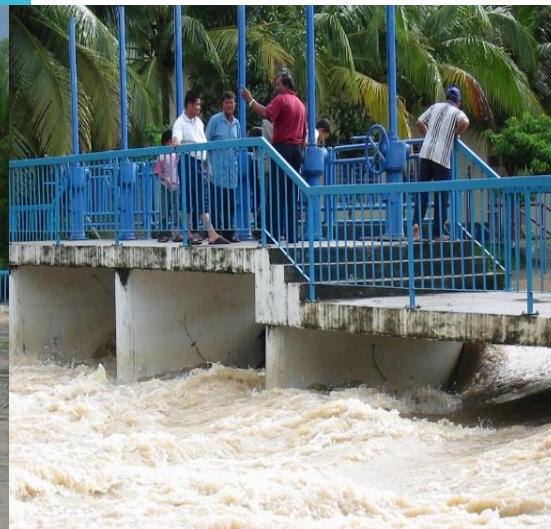
Overtopping due to floods (13 August 2003)
