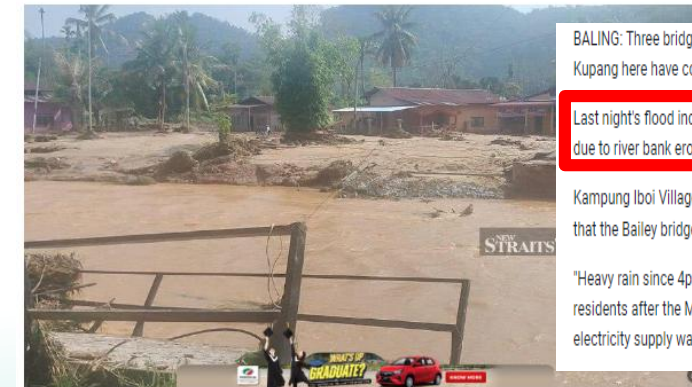
One of the bridges connecting residents of Kampung Iboi and Kampung Padang Empang along Sungai Kupang collapsed due to intense flash floods last night. - NSTP/AHMAD MUKHSEIN MUKHTAR
