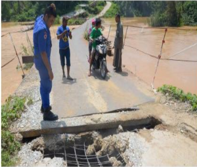
A temporary access bridge connecting Dabong to Gua Musang had to be closed due to several damages caused by heavy rain on Thursday. Pix by Ramli Ibrahim
