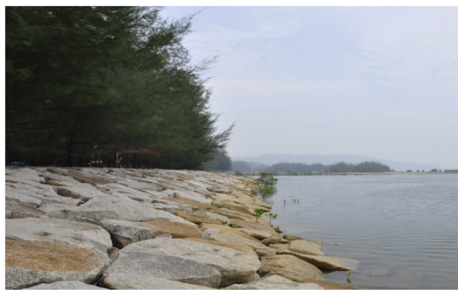
Fig. 8. Rock revetment at Taman Gelora, Pahang.
