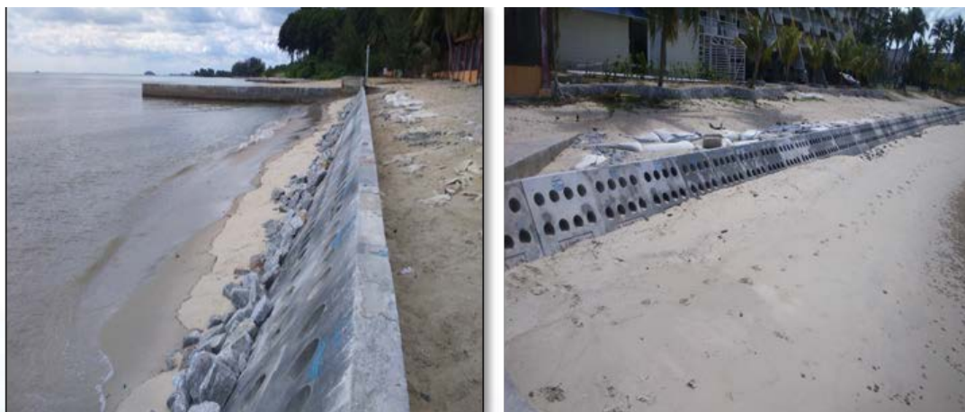
Figure 14: Condition of at Site A during extreme event (exposed toe) and calmer period (accretion of sediment)
