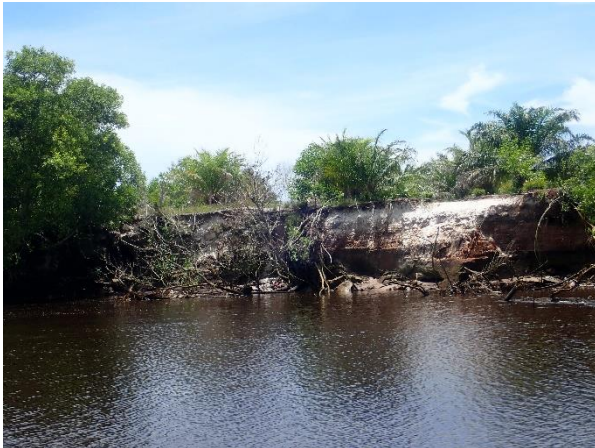
Figure 36: High erosion of river banks and also associated with died plants and trees
