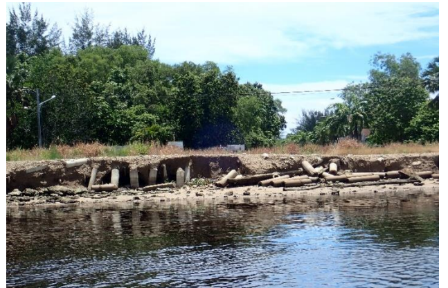
Figure 99: Very worst erosion near to river bank and vulnerable to district roads
