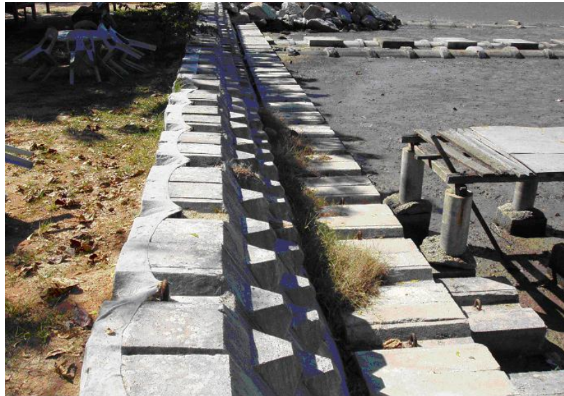
Figure 2.27 : Second Generation of Labuan Blocks as sloping “mattresses” at Taman Robina, Seberang Perai Utara, Pulau Pinang (source : DID, 2009)
