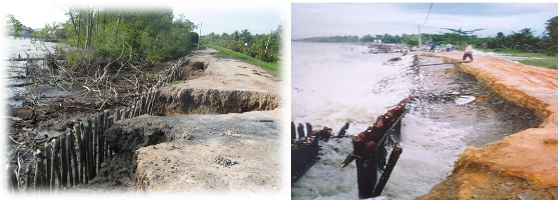
Figure 2.10 : Some example of damaging coastal earth bunds in agricultural area caused by wave attack (source : DID, 2009)
