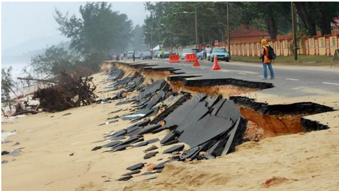
Figure 2.3 : Severe coastal erosion occurred in Teluk Lipat, Dungun, Terengganu just after the North-East Monsoon due to the destructive wave action.
