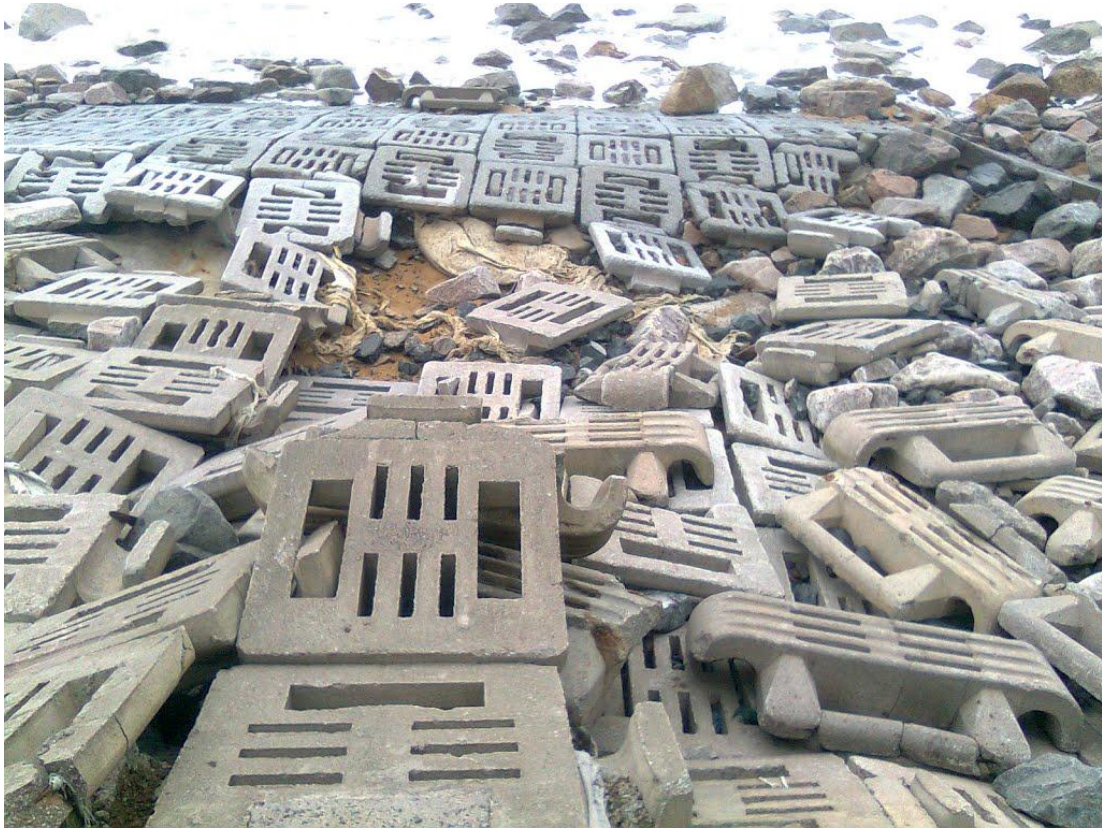
Figure 2.15 : The failure condition of interlocking flex-slab revetment after being hit by big waves at Pantai Teluk Lipat, Dungun, Terengganu (source : DID, 2009)
